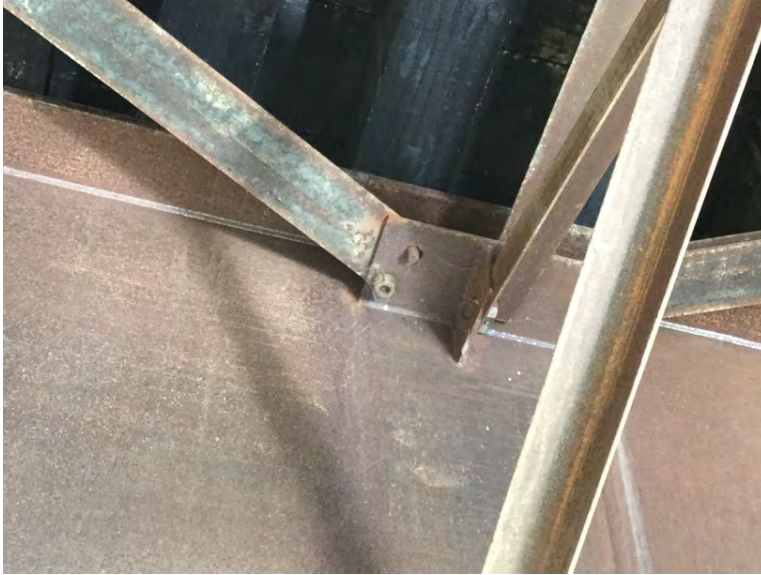
Missing bracing nut
